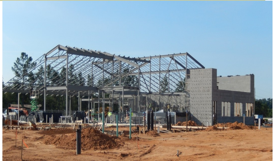
The steel supports are going up very quickly as the new lab structure begins to take place.
